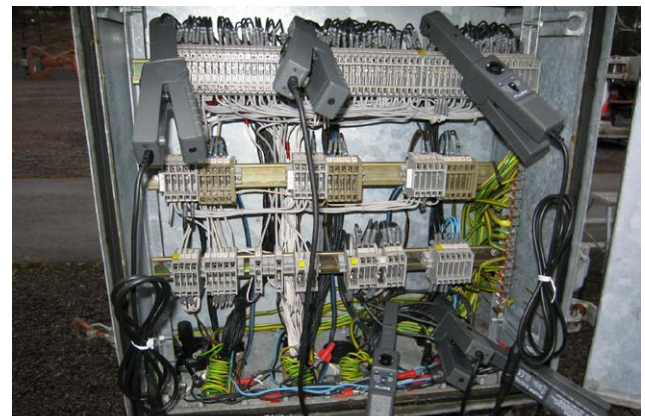
Figure 3 Control cabinet with current clamps
