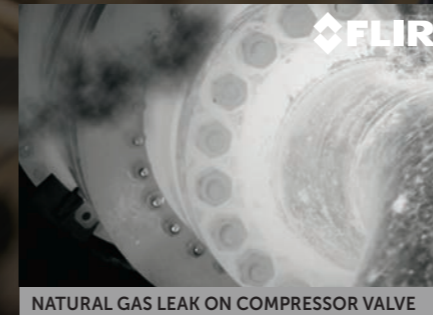
NATURAL GAS LEAK ON COMPRESSOR VALVE
