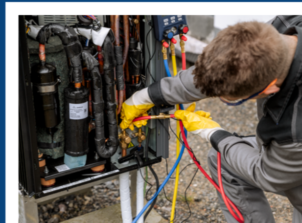
Easy to carry out maintenance work on heat pumps.
