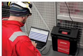
3 Diagnostic partial discharge testing
